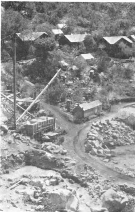
SITE OF THE POWER-HOUSE AND CAMP OF THE J. G. WHITE ENGINEERING CORPORATION
