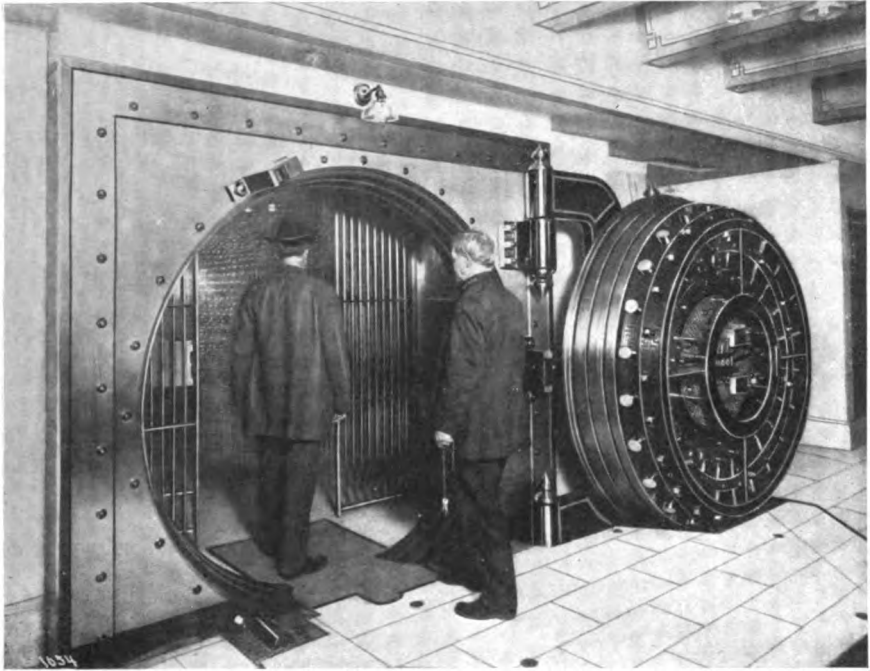
SAFE DEPOSIT VAULT AMERICAN TRUST AND SAVINGS BANK, BIRMINGHAM, ALA.
