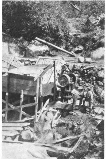
CONCRETE MIXER AND ROCK CRUSHER PLANT AT THE LOWER END OF TUNNEL NO. 12
