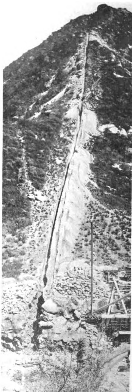
EXCAVATION FOR THE PENSTOCK FROM THE TOP OF PIPE LINE HILL TO THE POWER-HOUSE SITE AT BASE OF THE MOUNTAIN
